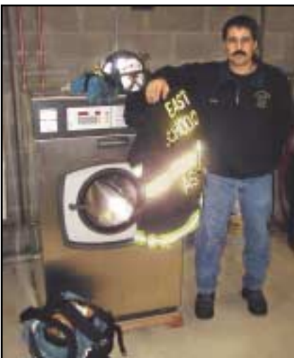
Assistant Fire Chief Steve Schweigert of the East Schodack Fire Company installed a Continental 30-pound soft-mount washer extractor—insuring that the department’s gear is getting cleaned properly and protecting his staff of 40 firefighters.
